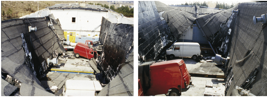
Fig. 1. Overview of the collapsed roofing construction.
