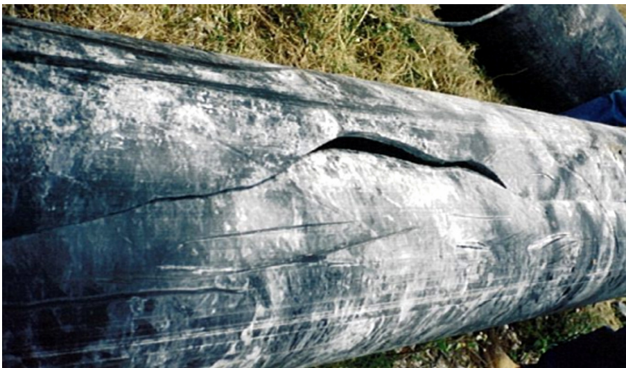
Fig. 1. Longitudinally cracked HDPE-tube.
