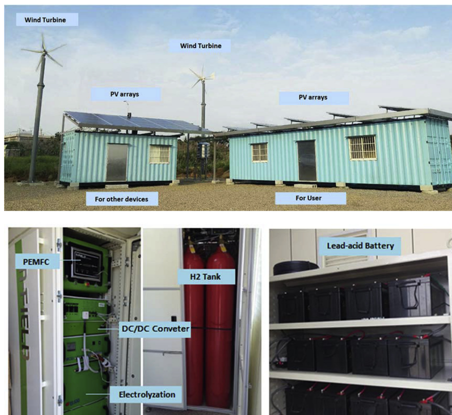
Fig. 1 – The CECI green building [14]. (For interpretation of the references to color/colour in this figure legend, the reader is referred to the Web version of this article).
