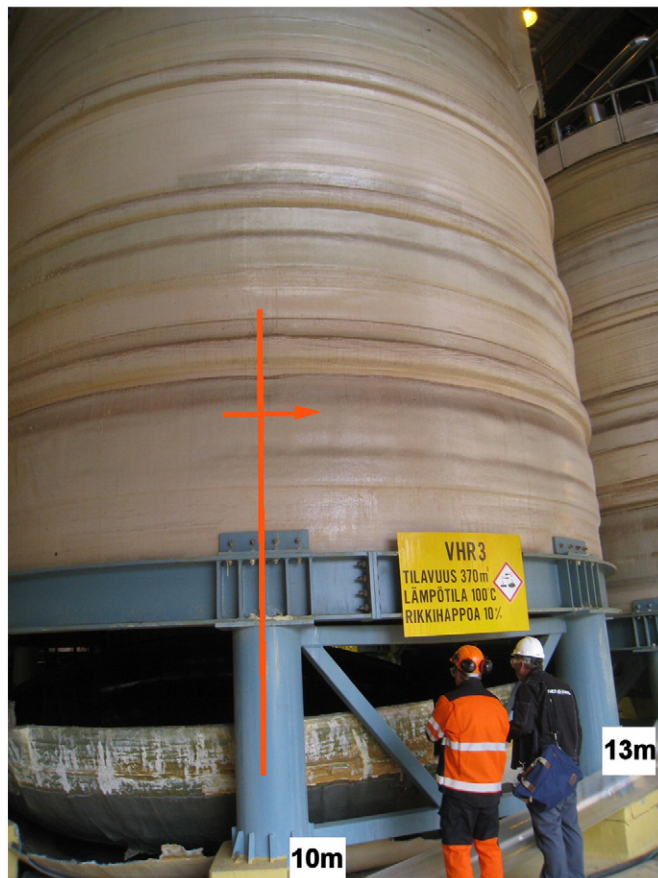
Fig. 1. Overview of the failed reactor.
