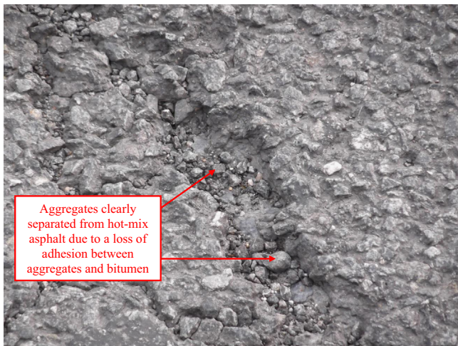
Fig. 1. Hot-mix asphalt that has suffered from stripping, as a consequence of a loss of adhesion between the aggregates and the binder due to the action of water.
