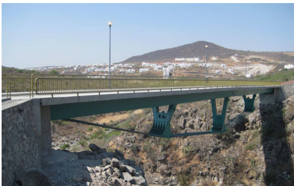
Fig. 2. San Miguelito creek footbridge in Queretaro (Mexico) designed by Carlos Fernandez Casado SL and completed in 2008. Photo courtesy of Arturo Perez Aguilar and Christian Balcazar Benitez (Mexpresa).
