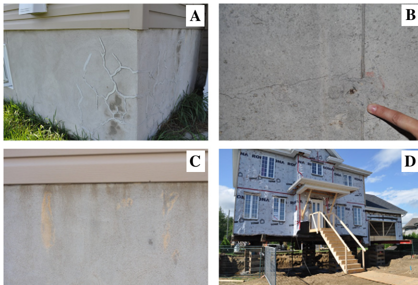
Fig. 1. Visual signs of concrete deterioration on the foundations of Trois Rivières private houses and the ultimate measure taken for replacing the affected structures: A) map-cracking filled with caulking material; B) pop-outs; C) discoloration; and D) total replacement of a concrete foundation.
