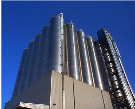
Fig. 1. Southwest corner of the silo group in the port of Antwerp (Belgium) where ovaling vibrations were observed in October 2002.
