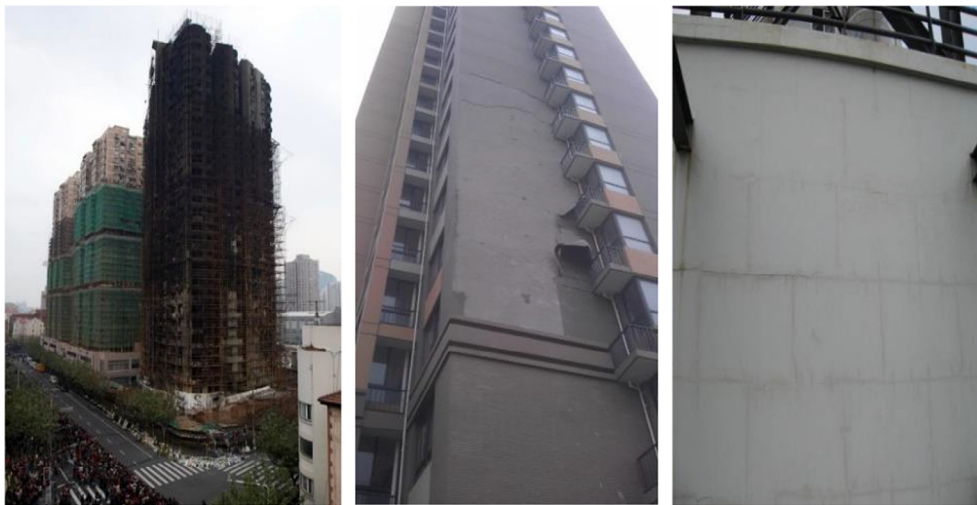
Fig. 1. Accidents for exterior thermal insulation system in Shanghai (fired, dropped, cracked).
