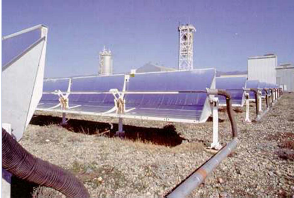
Fig. 1. ACUREX distributed solar collector field.
