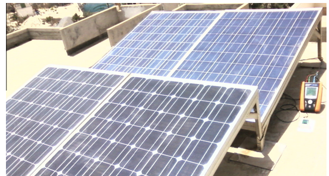
Fig. 1. Photovoltaic test field at Dakar in Senegal.
