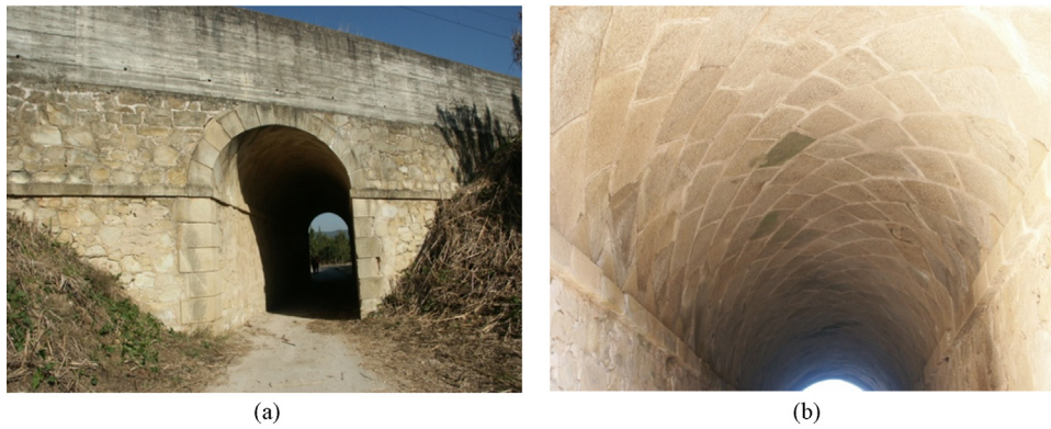
Fig. 1. Typical skew masonry arch constructed using the English method: (a) front view and (b) detail of the intrados.
