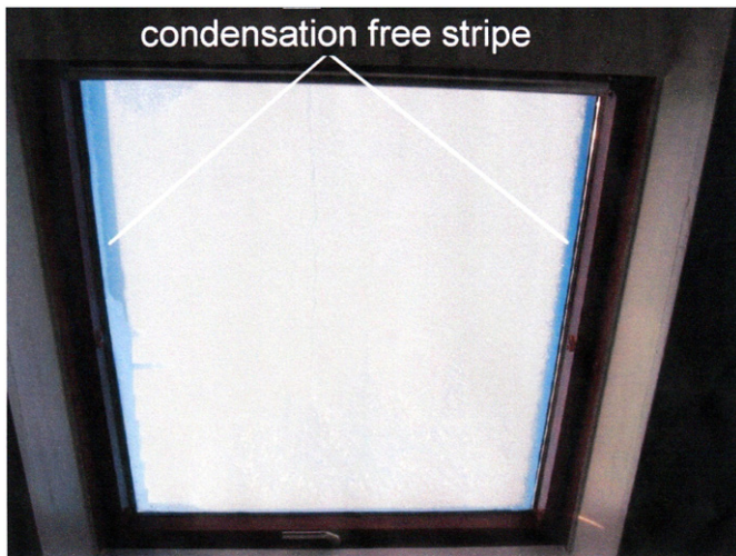
Fig. 1. Skylight glazing with frost on the outside surface.
