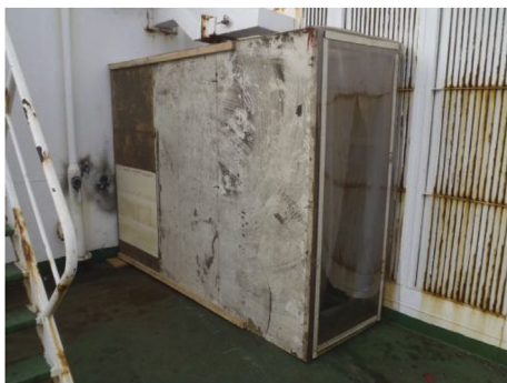
Fig. 3. The cabin containing asbestos.
