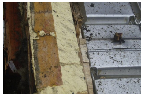
Fig. 6. The position requiring heat insulation often uses solid foam in the ship.
