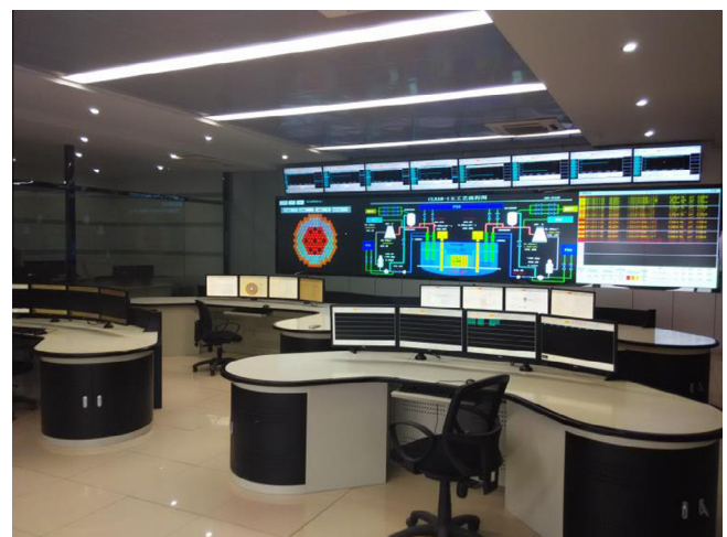
Fig. 2. Main control room of ADS-CLEAR simulator.
