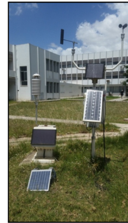
Fig. 2. Meteorological station energy systems of the National Institute of Meteorology of Tunisia.
