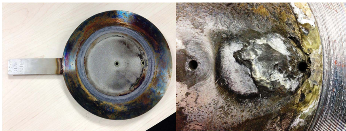
Fig. 1. Photo of the back-pressure orifice plate installed at well XH-01. The orifice plate is 10.16 cm (4 in.) in diameter. Right photo shows the enlarged view of the damage near the drain orifice.
