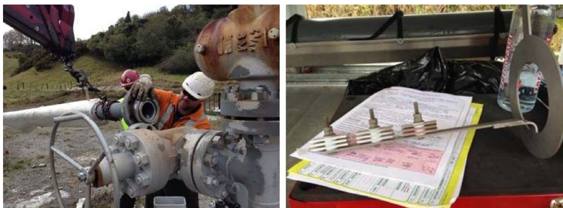
Fig. 2. CL900 RTJ Flange (left) where the corrosion rack (right) was installed.
