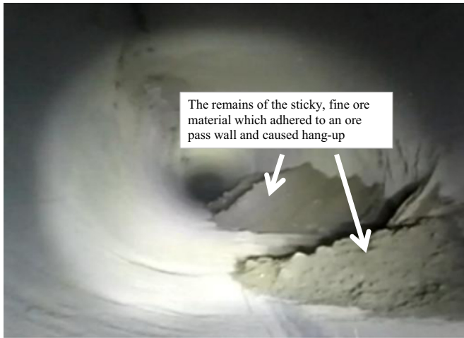
Fig. 1. The photograph shows the inside of an ore pass (looking down) once a hang-up had been dislodged by intervention. The remains of the sticky, fine particles which adhered to the ore pass wall are clearly visible. The ore pass is circular in section with a diameter of 2.8 m and is inclined at 70° above the horizontal. The ore contains particles as large as 1.2 m, although larger particles do not adhere to the ore pass wall so they are not present in the photo.
