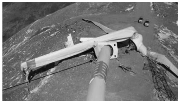
Fig. 2. Collapsed wind turbine tower in North Bridge wind farm in Guazhou, Gansu.
