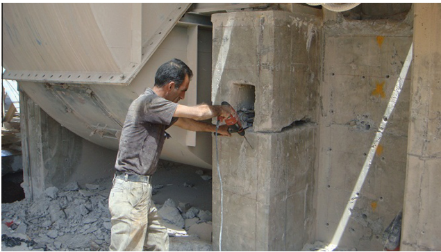
Figure 1 Typical concrete foundation of induced draft fan systems in which cracks occur.
