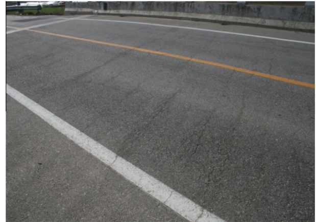
Fig. 1.2. Pavement cracks of an in-use GFRP deck (Gae-Jung Bridge).
