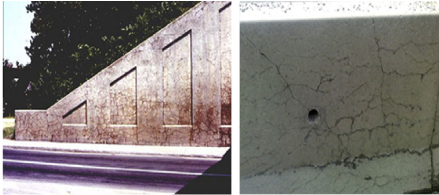
Fig. 1. Severe map cracking on the wing wall of 30 year old bridge structure affected by ASR [2], Highway Protection Barrier [3].
