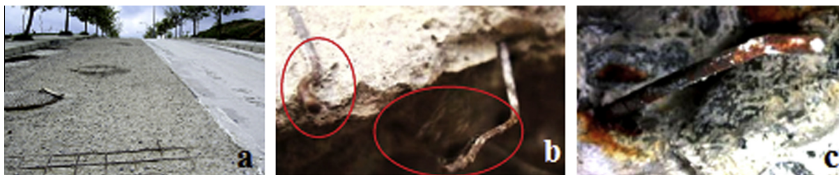
Fig. 1. The expose to negative condition of steel fibers and rebars in concrete.
