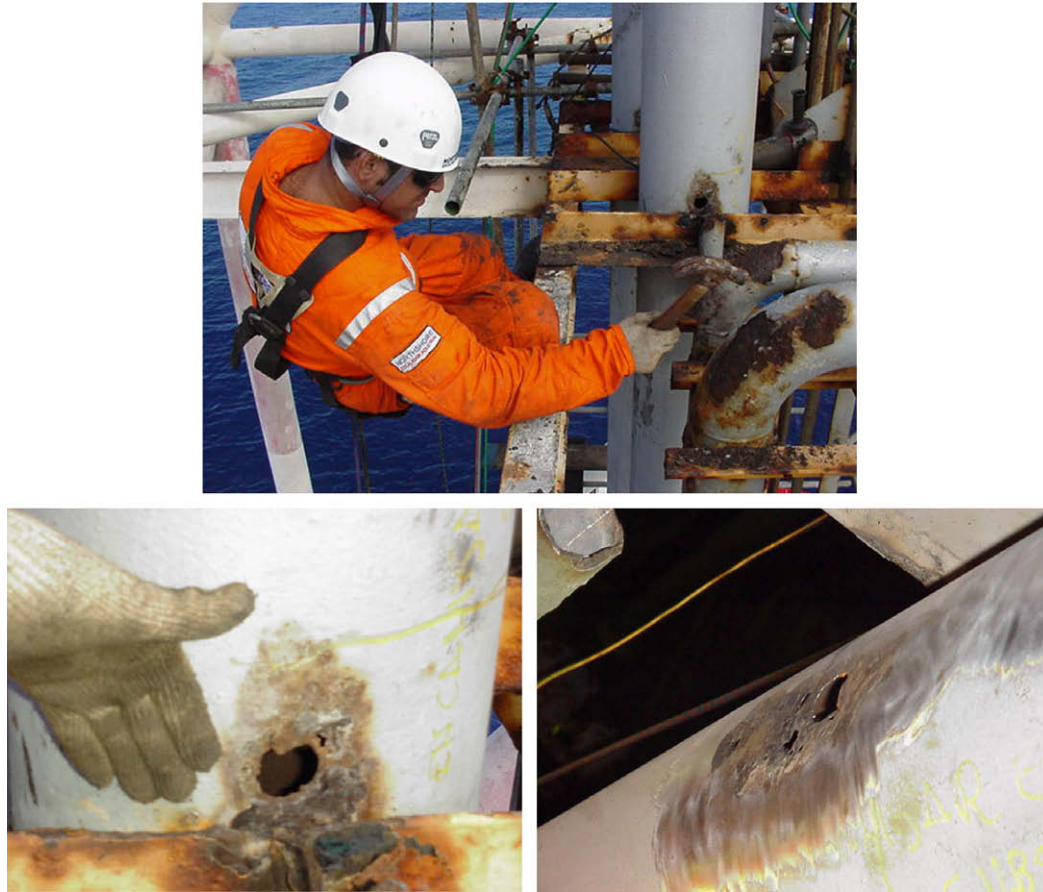
Fig. 1. Corrosion damage in produced water pipelines.
