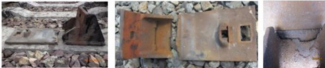
Fig. 2. Typical picture of destruction of counter rail bearing plates.
