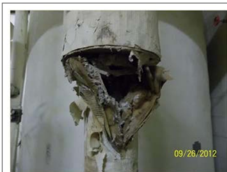
Figure 3: Asbestos thermal system insulation deterioration, Lexington, VA, 2012
