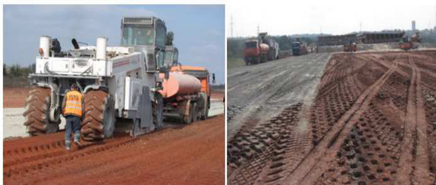
Figure 1: Construction of a highway bypass round Donetsk in the direction of Zaporizhzhia
