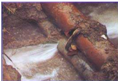
Fig. 1. Leaking sewer pipe next to a leaking water pipe (Karim et al., 2003)
