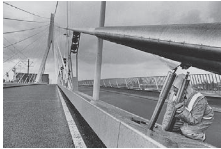
Fig. 1: Used new dampers to the Erasmus bridge to prevent vibrations. Photo: courtesy of TU Delft.
