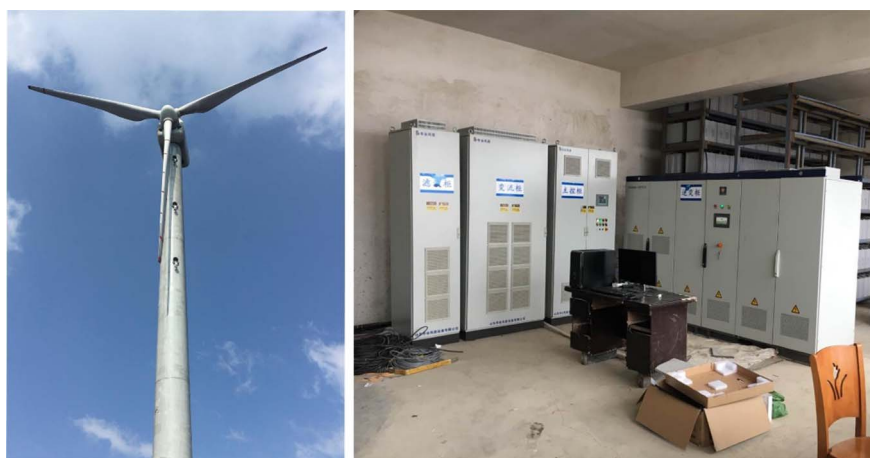
(a) 300kW wind turbine and control room.
