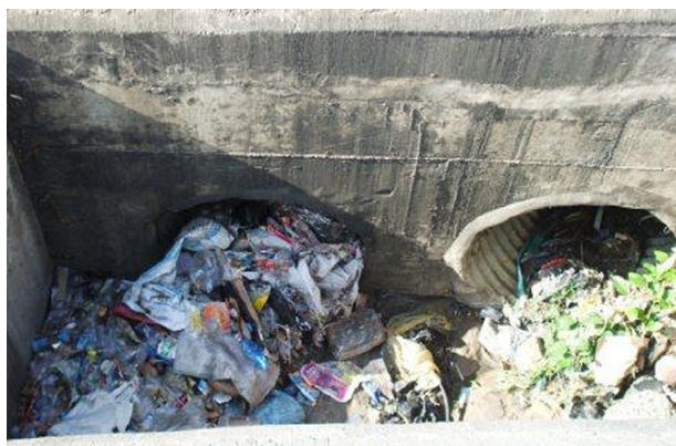
Fig. 1. Photographs showing waste plastics including water sachets blocking urban drainage in Ghana.
