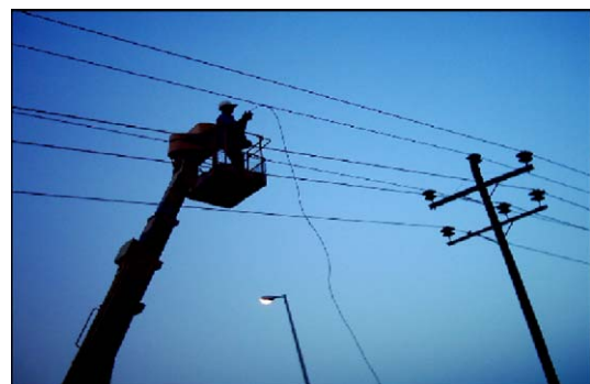
Fig. 3. Connection of a conductor to one phase.
