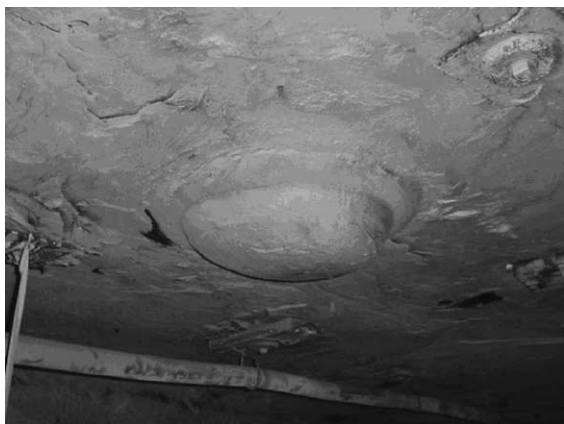
Fig. 1. Typical nature of carbonate nodule exposure in the immediate roof. Note what appear to be concentric compaction rings in black shale around the nodule, and slickenlines that are vertical and longitudinally arrayed on the nodule surface.
